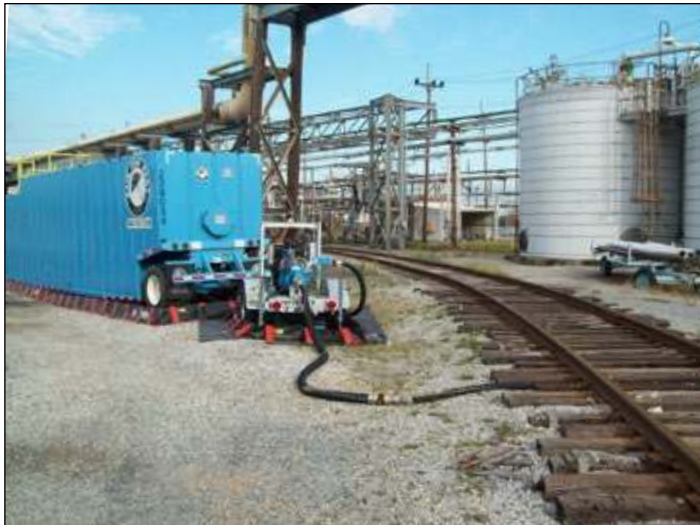
Rain for Rent provided the network of equipment needed for all 29 job sites needed in the industrial plant turnaround project.
