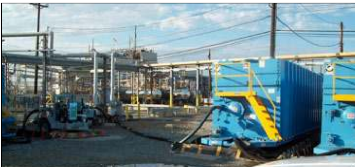
Auto start capabilities and visual alarm agents were utilized at some sites to automate sections and reduce spill risks.
