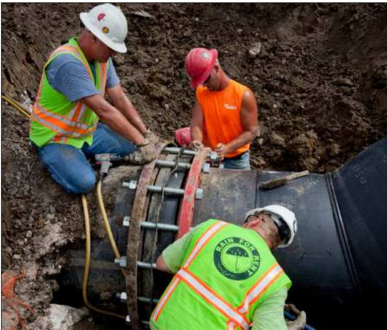
A section of 42 inch HDPE discharge line for pump station 2 is bolted in place. This line was fed by a FP-1050 capable of 68,500 gpm.
