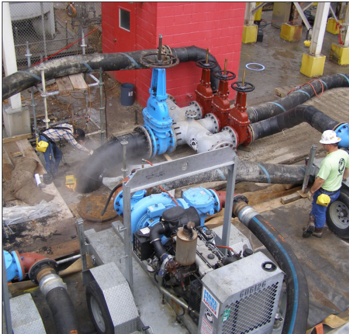
DV200c pumps, HDPE pipeline and hoses provided 24-hour bypass pumping to keep the pulp mill operational
