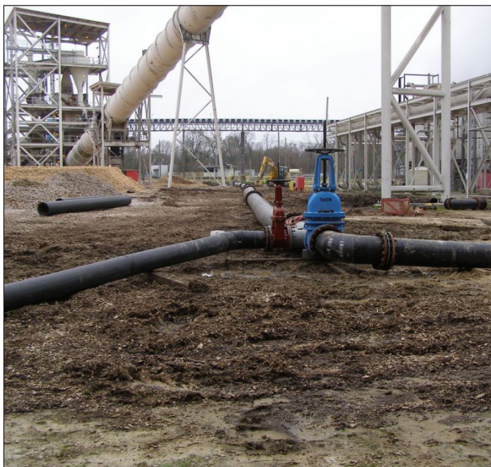
All pump stations were monitored 24/7 to keep the mill online.
