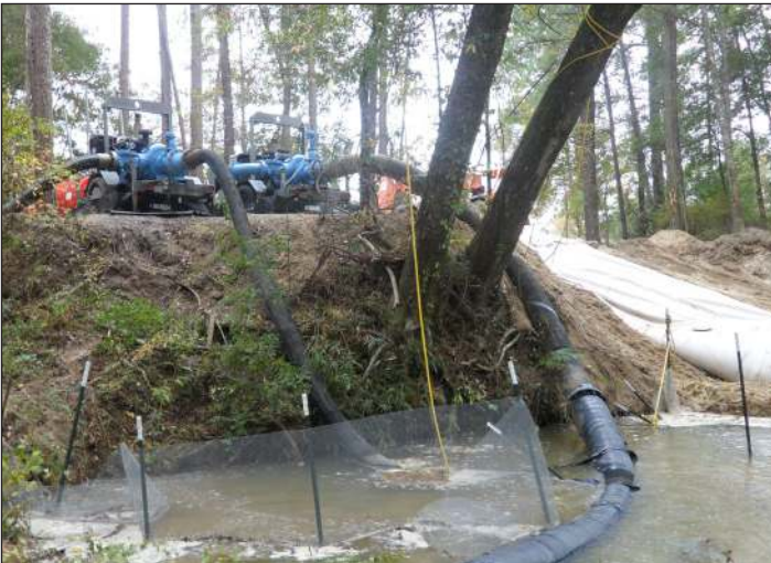
The multi-phase filtration system allowed creek excavation to proceed without the cost of transporting contaminated water.
