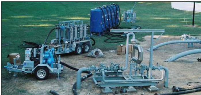
The filtered water met all standards for discharge in a nearby creek.
