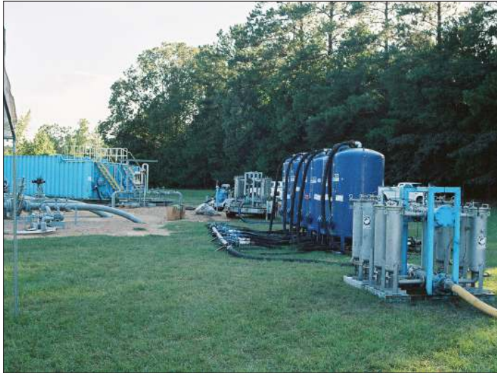
A filtration system using 10 micron bag filters and carbon filters proved cost-effective for hydrotesting company.
