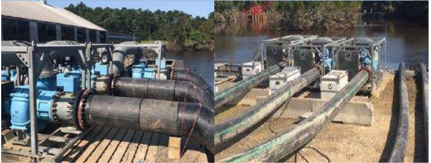
Three pumps created a 100,000 GPM system to bypass the primary pump station during flood repairs.
