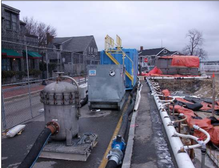
Dewatering was crucial for the correct installation of a solid foundation for the new five-story New England theater.
