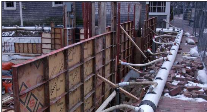
Four months of continuous dewatering to a depth of 18 feet provided stability and a dry work environment.
