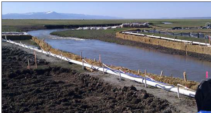
As temperatures rose the boring operations passed under a small river, before they are secured on the barge.
