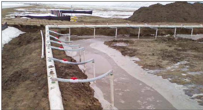
Six weeks of continuous dewatering and below freezing temperatures made the job a challenge.
