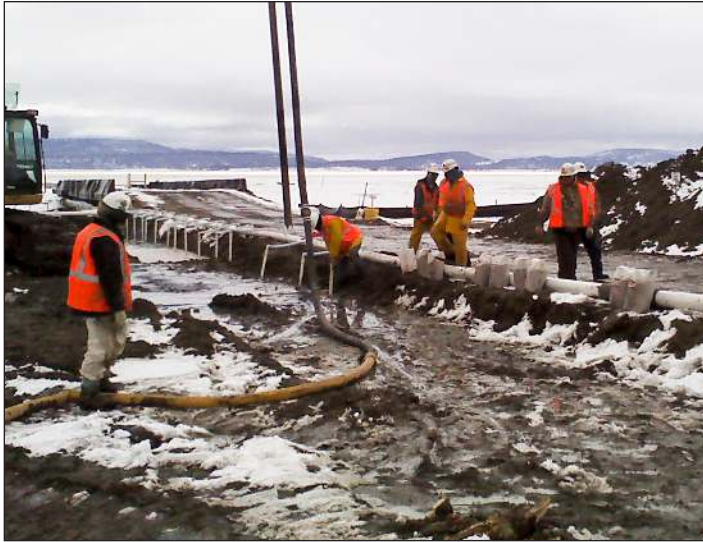
One of the two 75-point wellpoint dewatering systems is installed in frozen ground in Southeastern Oregon.
