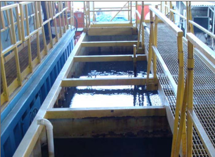
Solids settled out in weir tanks with the aid of polymer injection.
