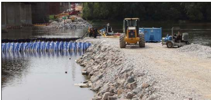
The multi-phased project overcame what the project manager called challenging environmental conditions.
