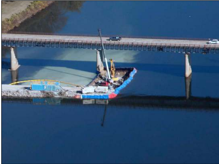
This aging bridge would be replaced, dewatering was needed to construct the pilings for the new structure.
