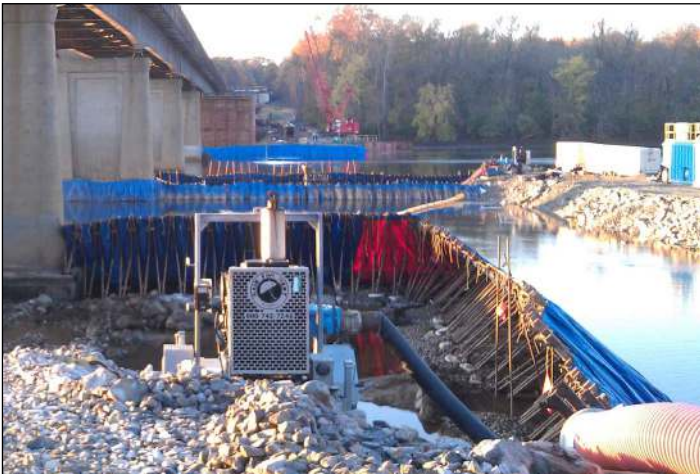
Portadam and Rain for Rent collaborated to provide dewatering and cofferdam services for the new construction.
