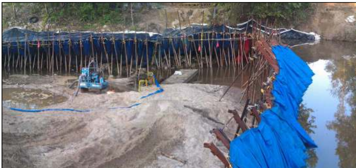
The project went from a standstill, at risk of delay to an on-time completion thanks to the partnership of Portadam and Rain for Rent.
