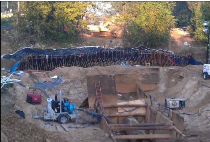
The gravity-fed river bypass flume helped to save the pipeline contractor money on pumping costs and project delays.
