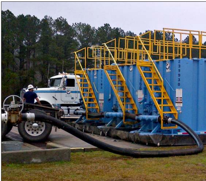
WORKSAFE™ Steel Frac Tanks were used to temporarily store the water produced from pigging a fuel pipeline at the air strip.
