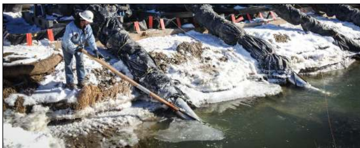
Rain for Rent's pump watch employees had to remain vigilant and break up ice blocks before it clogged pump suction lines.
