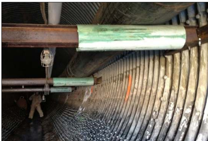
To allow the bypass to be routed under the airport, the HDPE pipeline was suspended on engineered bracing.
