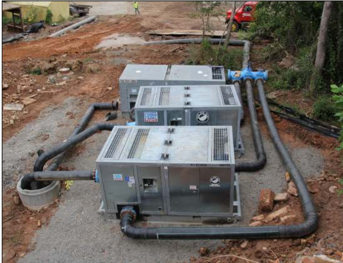
Sound attenuated pumps were used to bypass sewer lines in residential areas, lessening the noise impact on the community.
