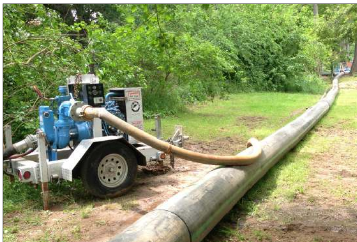
For more than a year, Rain for Rent worked directly with contractors to manage up to 20-MGD of sanitary sewer bypasses.
