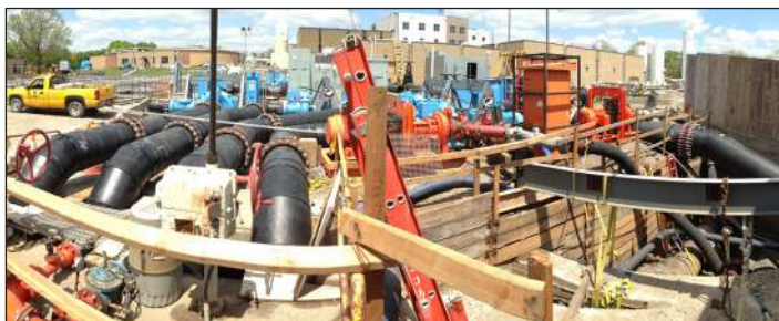
The automated electric-driven bypass system used four stages of pumps to scale to dewatering needs.
