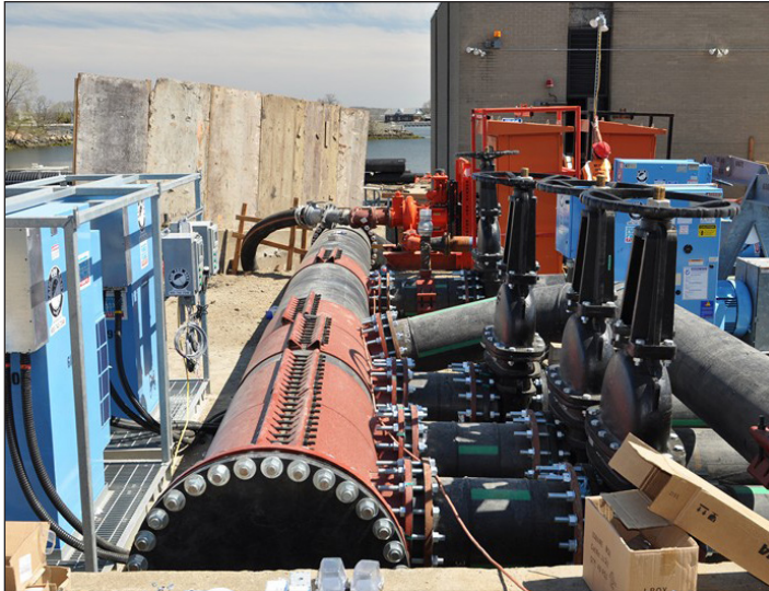
Variable Frequency Drives powered the DV400 pumps, allowing them to throttle up and down based on water levels in the pit.
