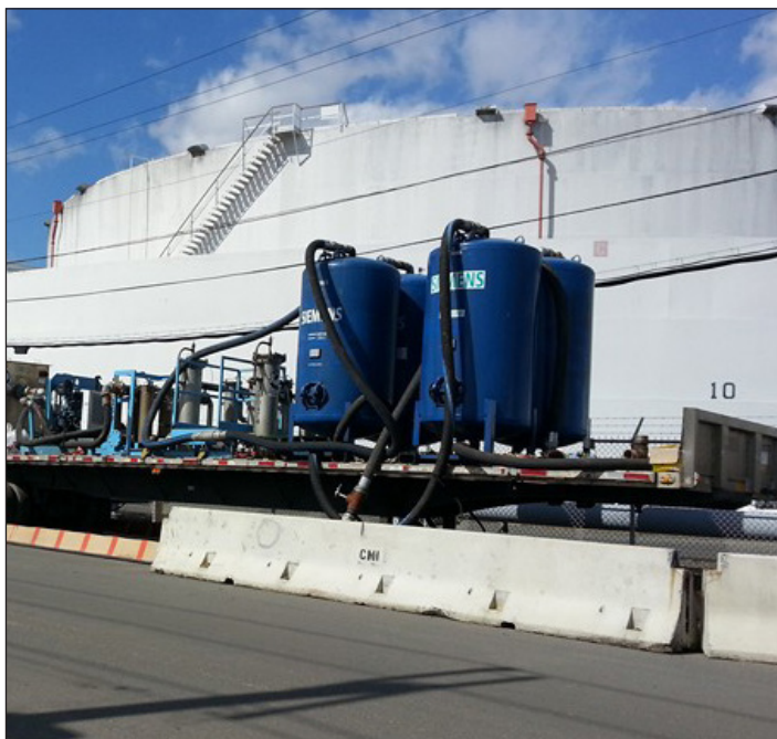
Pumps, oil water separators, bag and carbon filtration provided 200 GPM of dewatering and filtration from each trailer-mounted system.
