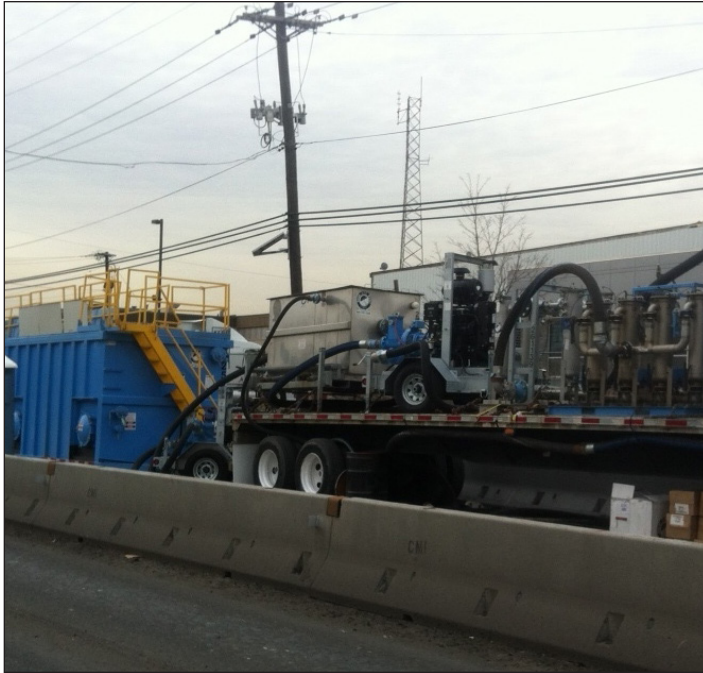
The dewatering and filtration system was staged on trailers to allow filtration to move as the tunneling project progressed.
