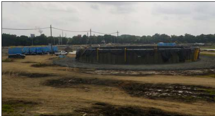
The LakeTank required a much smaller footprint than equivalent liquid storage in frac tanks, and allows vacuum trucks to siphon off any oil.
