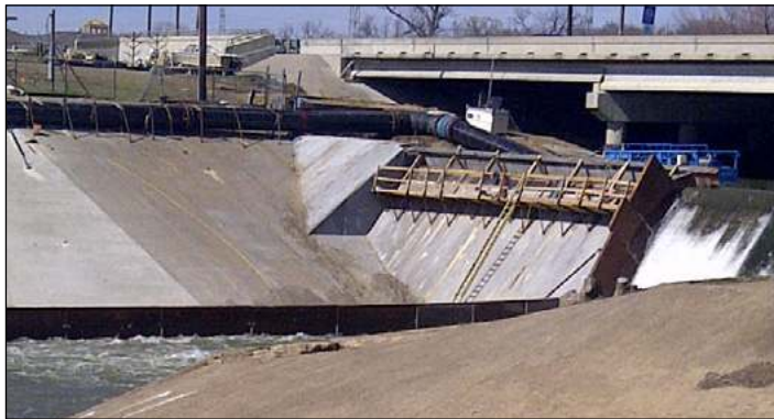
The cofferdam used by the rehabilitation contractor worked with the floating pump to provide conditions needed for repair work.
