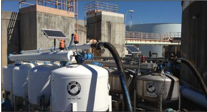
The water treatment plant needed a filtration system bypass so they could repair their treatment plant in a week and a half.
