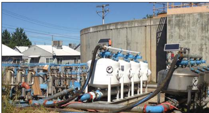
The system was designed to remove particulates to achieve a 0.3 NTU water clarity level.
