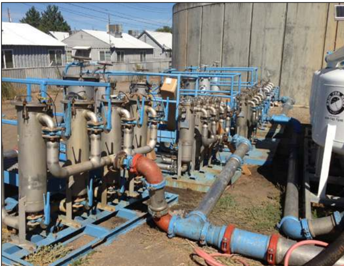
A combination of bag filters and sand media filters were used to polish the water.
