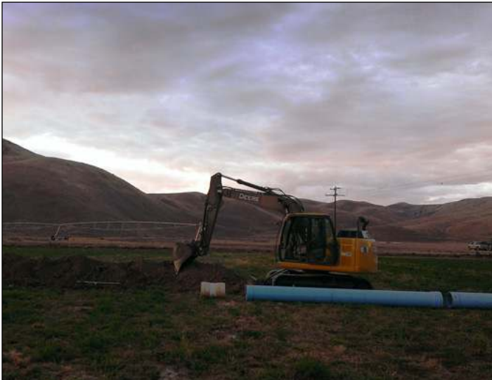
50,000 feet of gravity flow pipelines were installed to bring water to the pivots, which achieved 50% water savings.
