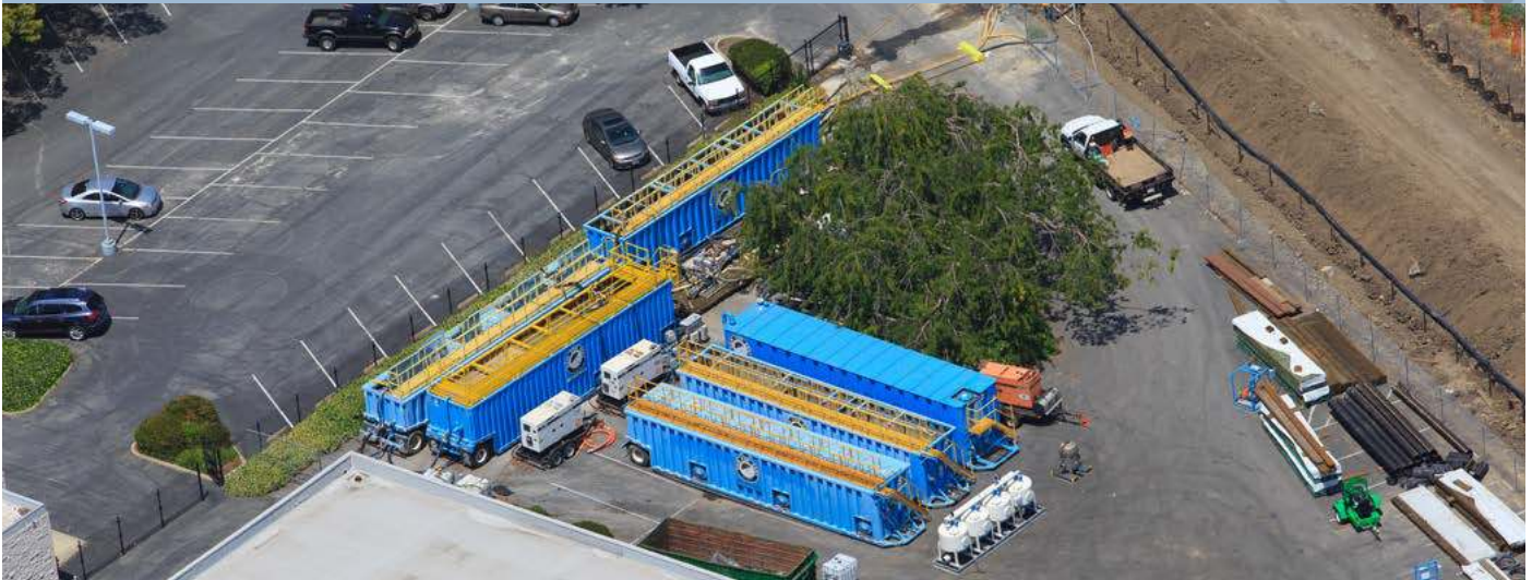
Dewatering Filter Train at Piper Ct., Milpitas CA.
