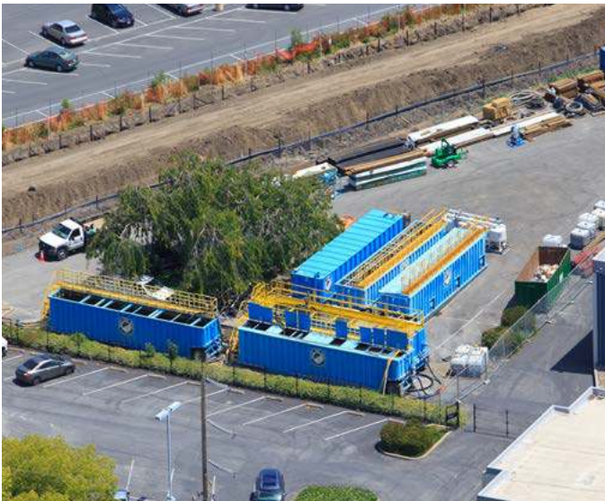
Dewatering Filter Train at Piper Ct., Milpitas CA.
