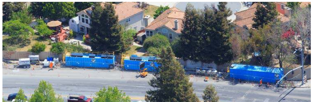
Filter Train at Montague for suspended solids.
