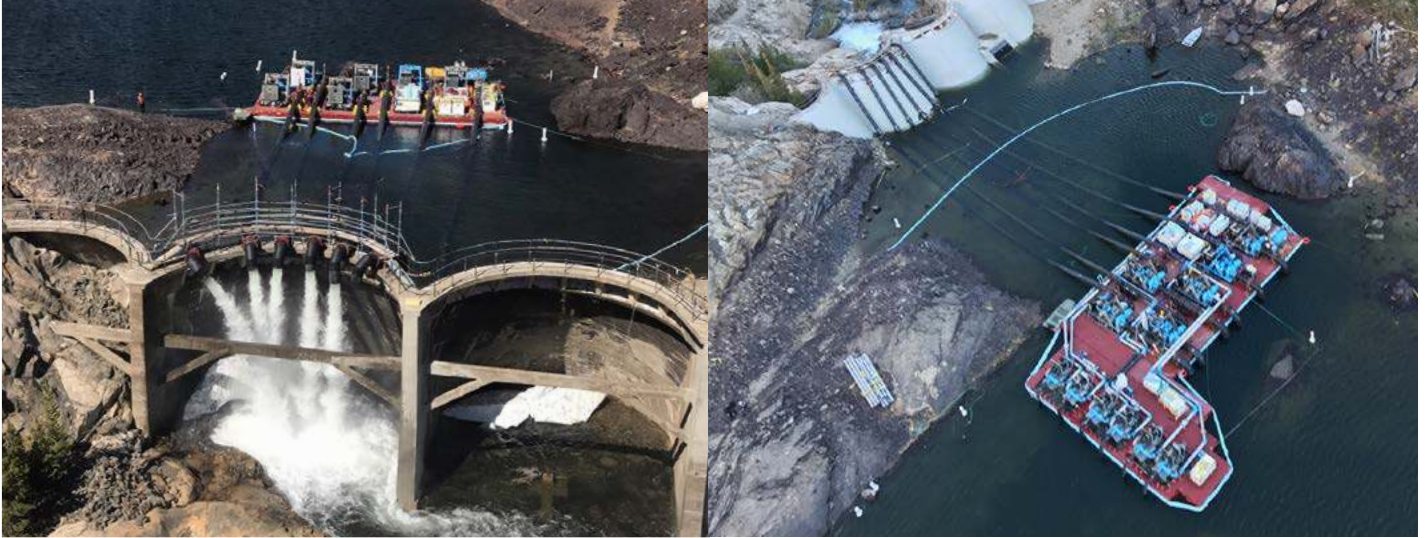
Twelve pumps removed 200 CFS of excess water from the lake to relieve pressure from aging dam infrastructure.
