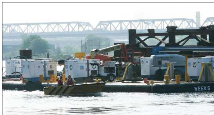
Dept. of Transit workers examine the DV-150 pumps before they are secured on the barge.
