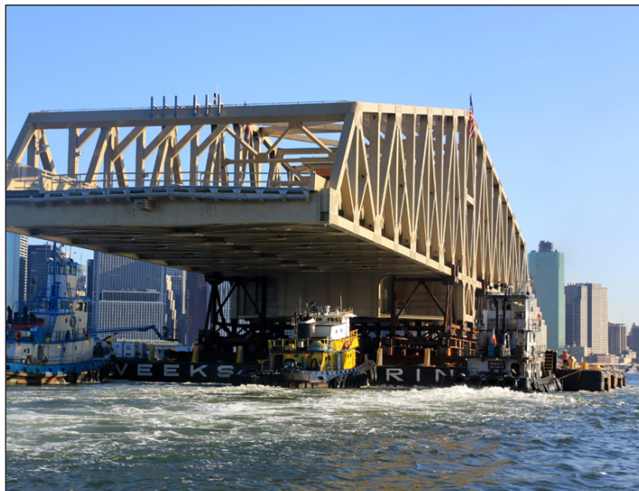
Three tug boats ferry the 2,400 ton bridge floating on a barge up the East River.
