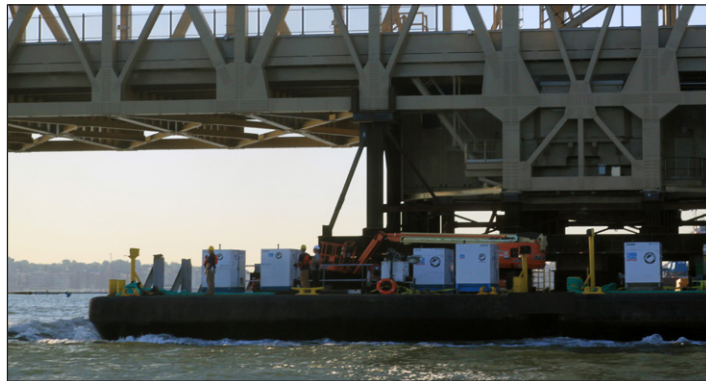
Precise level control was needed and DV-150 pumps were used to manage ballast levels on the barge.
