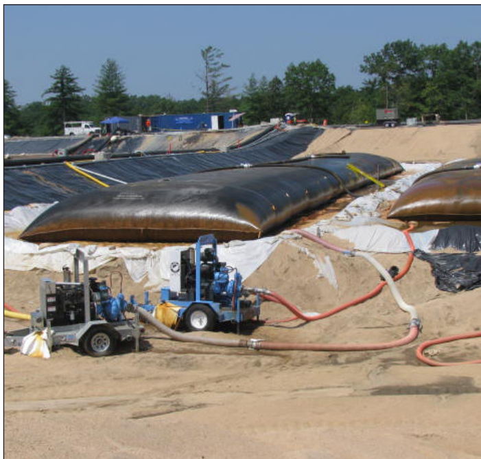
To prevent seepage, Rain for Rent pumps take effluent from geo tubes for finer polishing of PCB sediment along filtration train.
