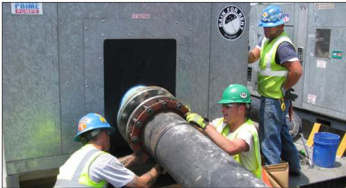
Rain for Rent installers secure HDPE pipe to the DV300i SA pump.
