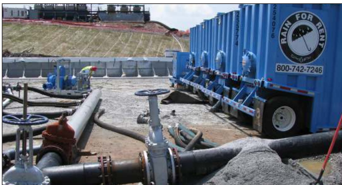
PCB-laden water was stored in steel frac tanks.
