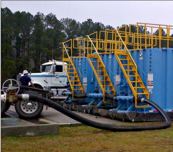
WORKSAFE™ Steel Frac Tanks were used to temporarily store the water produced from pigging a fuel pipeline at the air strip.
