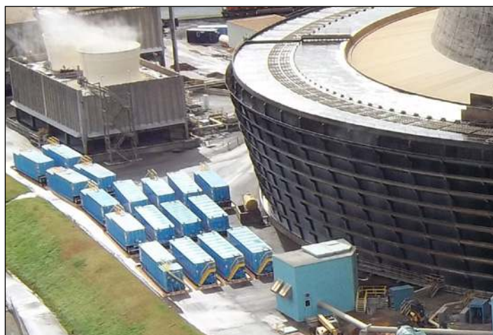
The hundreds of thousands of customers relying on this plant for power meant that every minute of maintenance counted.
