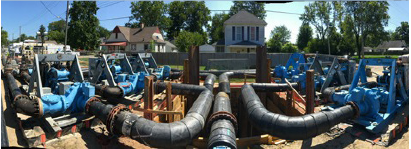
Six 18" pumps created a temporary pump station to bypass the sewer-flow through four 24" HDPE lines.
