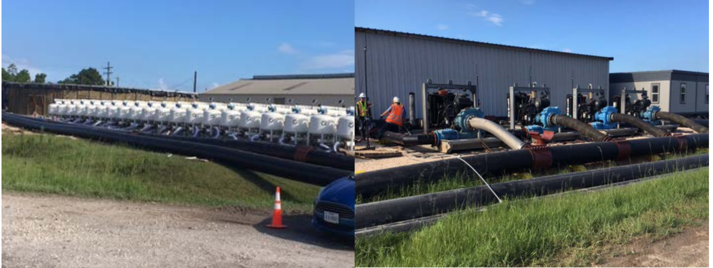
Water pumped through 20 sand filters, into a 3 acre-feet storage LakeTank® for a temporary water conveyance system during mill repairs.
