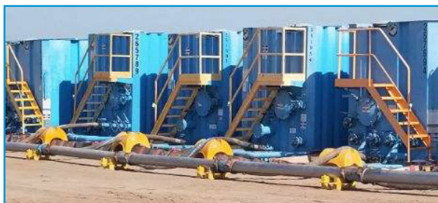
Manifold systems for bulk loading/unloading into frac tank batteries
